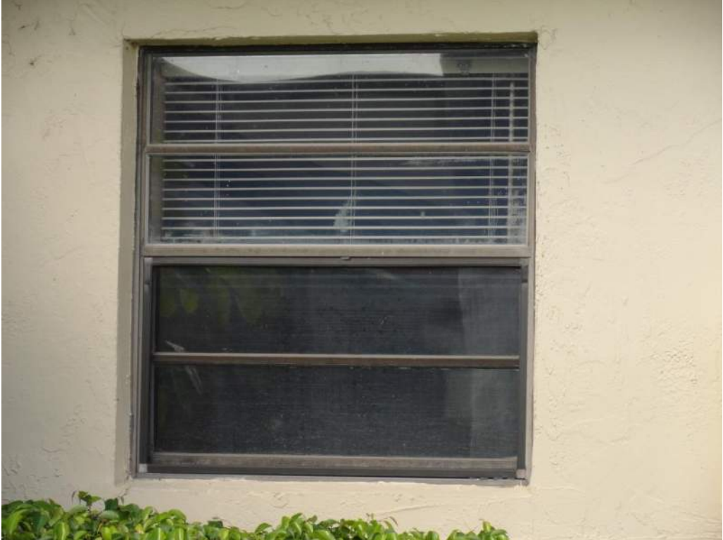
7. Opening Protection – Unrated Unprotected Windows
