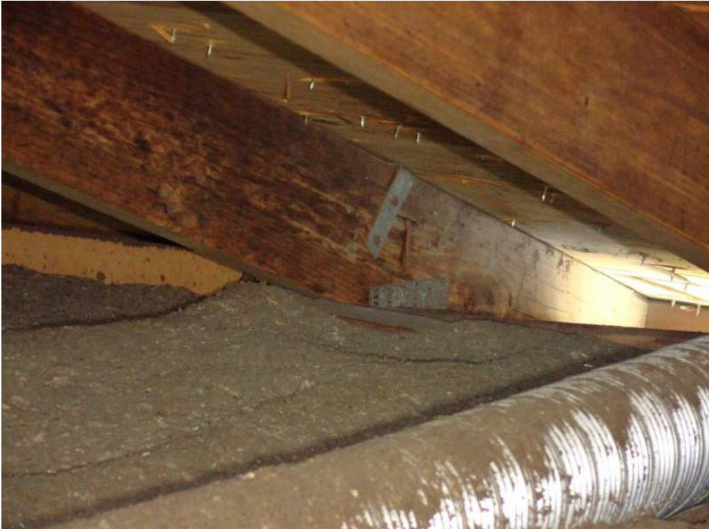
4. Roof to Wall Attachment – Single Wraps – Steel Straps w/ 1 Nail Min. at Back
