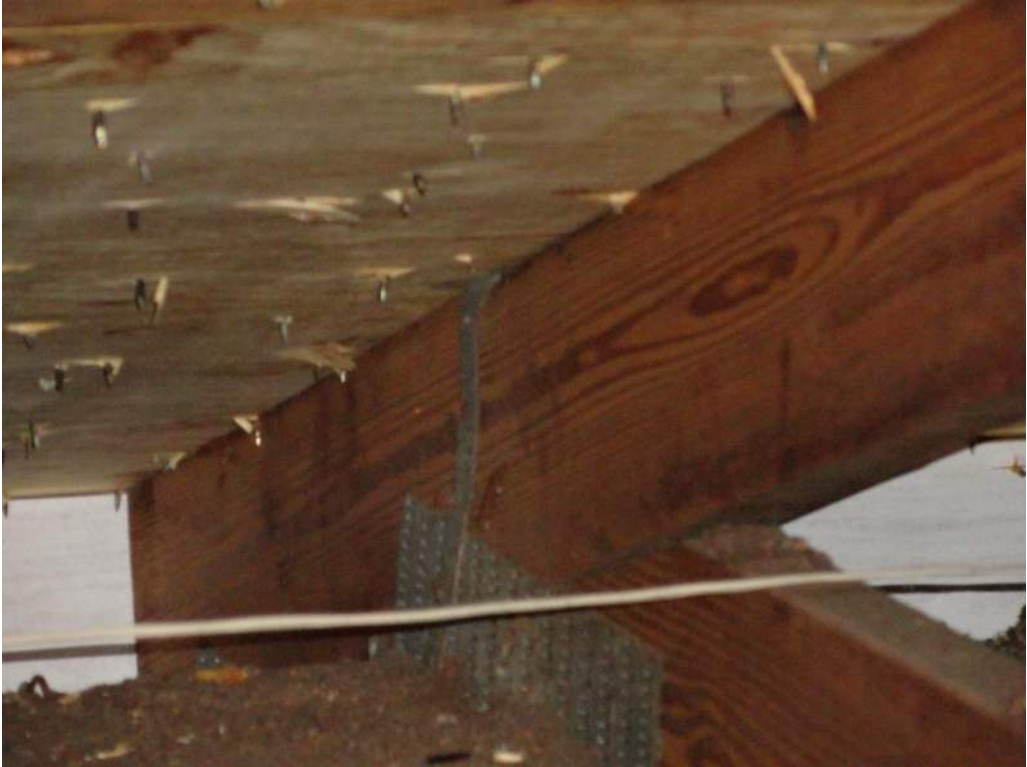
4. Roof to Wall Attachment – Single Wraps – Steel Straps w/ 2 Nails Min. at Face
