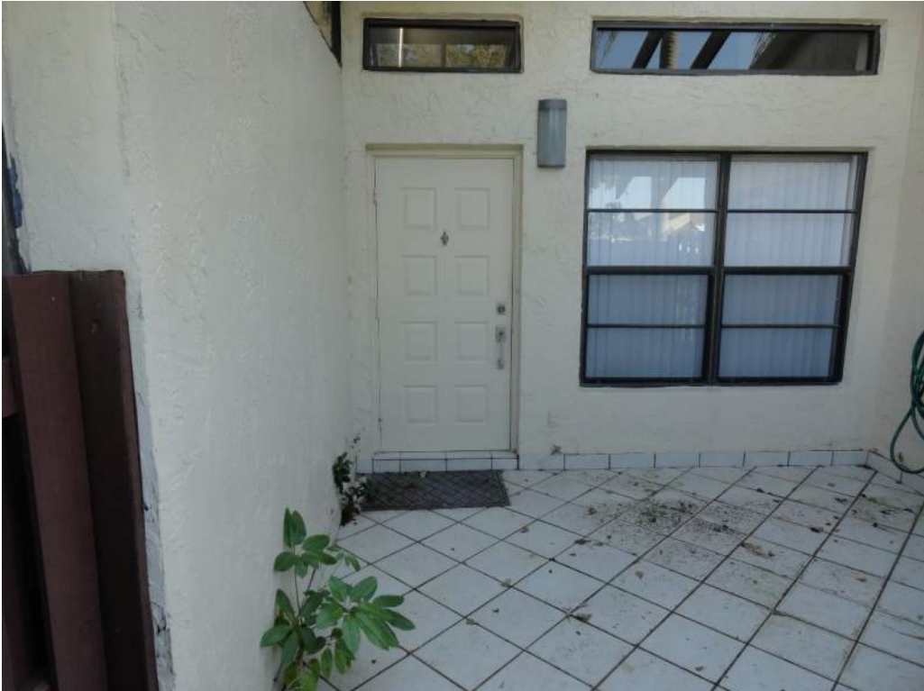
7. Opening Protection – Unprotected Unrated Unglazed Entry Door
